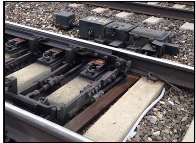
M-3 Switch Machine on Concrete Ties
